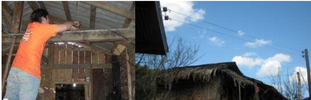
Figure 4: (Left) Showing old wires hanging loose (black) and new wires (grey) neatly pinned against beam. (Right) New household connection from power poles, using suspension clamps and steel rack
