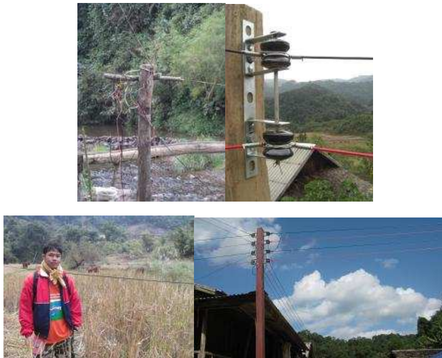
Figure 3: (Left Top & Bottom) Examples of previous bad wiring. (Right Top & Bottom) New wires provide a much safer and reliable system
